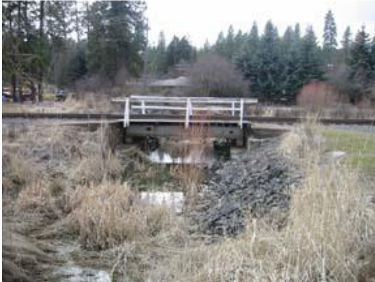
Figure 26: UPRR Bridge about 1/8 mile upstream of Bowdish road. Looking at upstream bridge face
