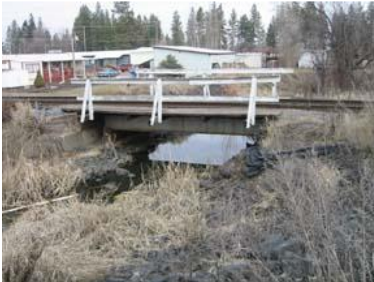
Figure 27: UPRR Bridge about 1/8 mile upstream of Bowdish road. Looking at downstream bridge face
