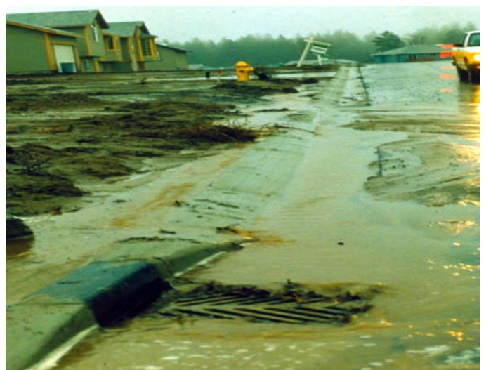
Figure 7. Construction Site Stormwater Runoff
