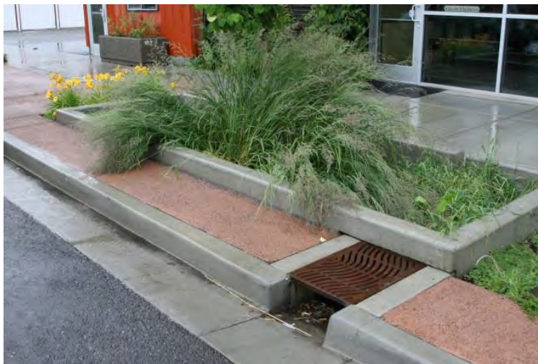
Figure 3-1. Example of a Bioretention area in the City of Spokane
