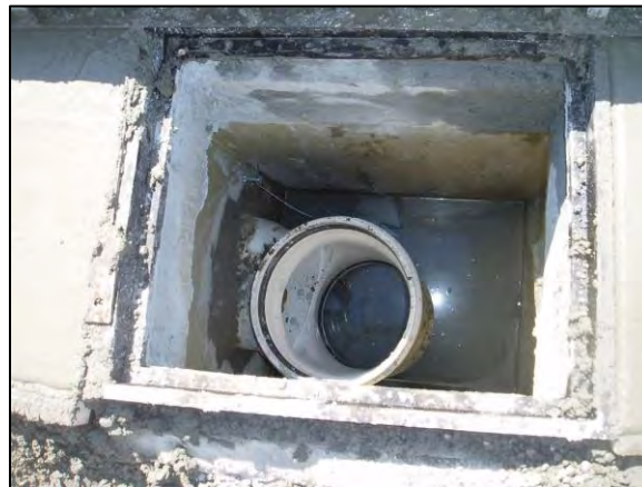
Figure 3-1. Spill control device: a standard catch basin with a retrofit (tee) on the outlet pipe
