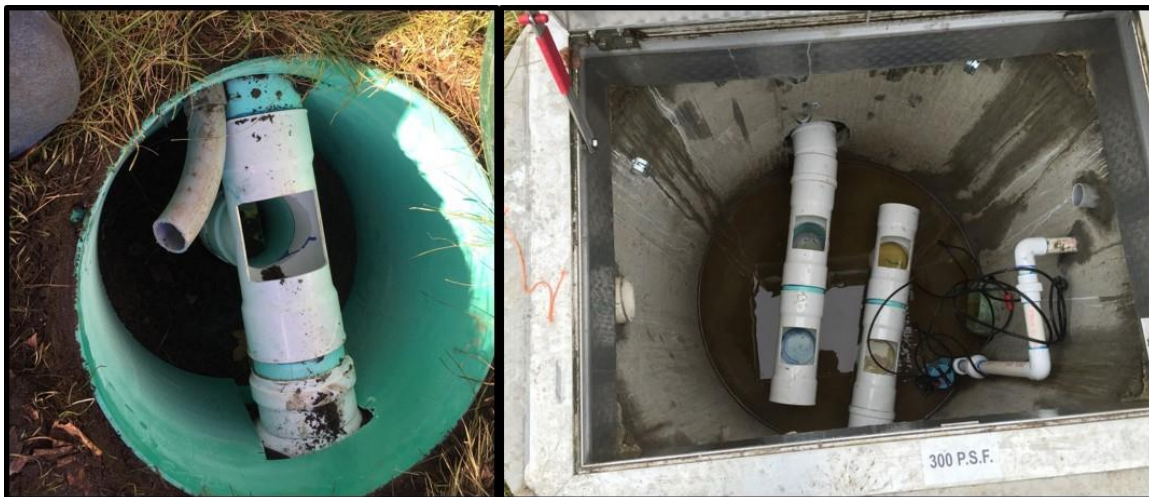
Figure 7.2 Influent sampling sump (left) and manhole-effluent sampling (right)
